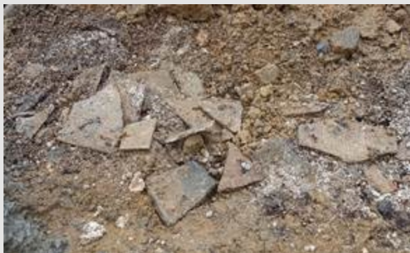
Asbestos Containing Material
