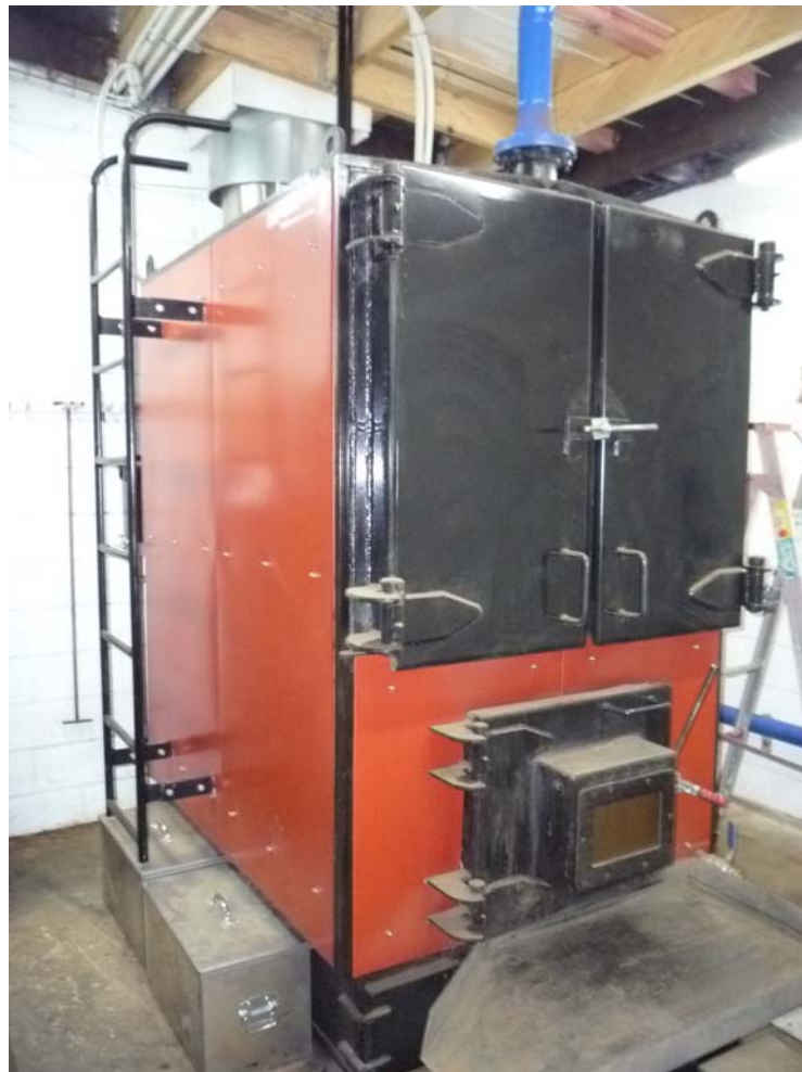
Matura Pool Boiler
