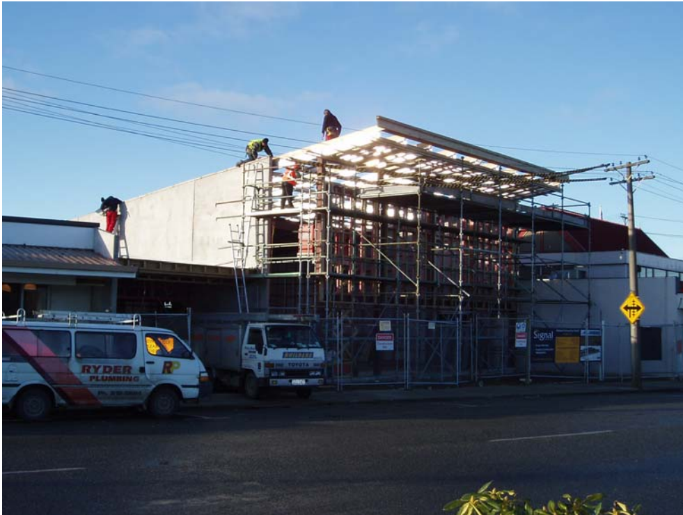
Mid August and the hall roof is nearly all on. All other roofs are completed.
